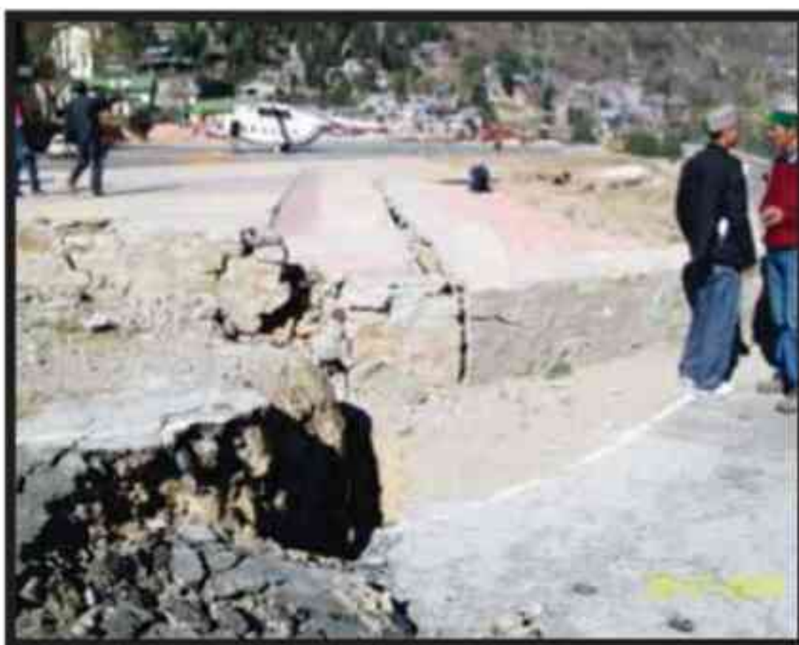
Reckong Peo Landslide
