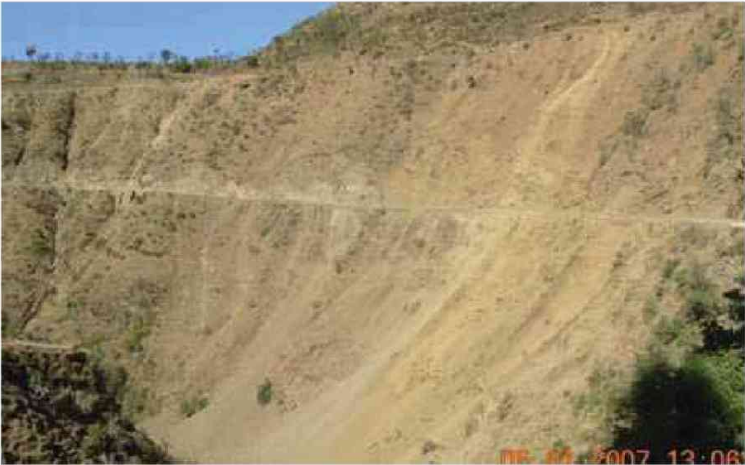
Photograph relating to Road Construction issues in hilly area
